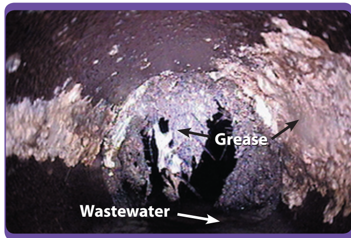
Image #4 – Grease stuck to the inside of sewer pipe
