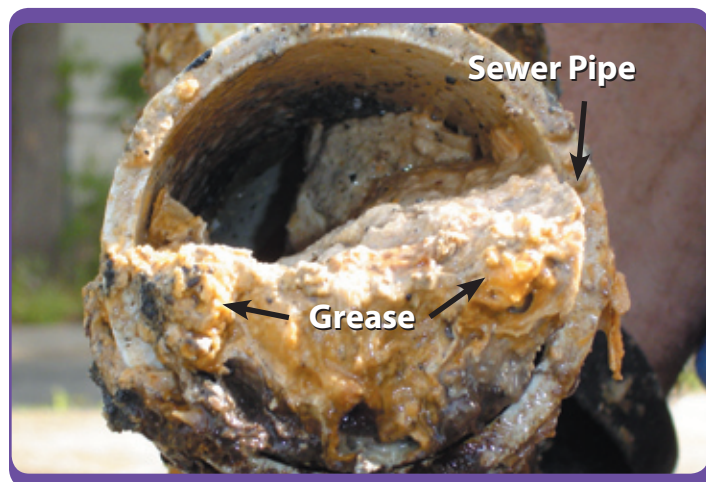
Image #3 – Grease inside of sewer pipe
