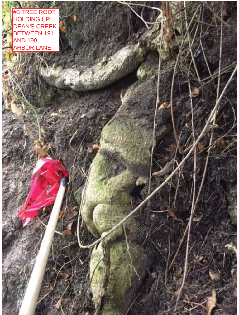
#3 STEEP VERTICAL DROP OF DEAN'S CREEK EROSION
