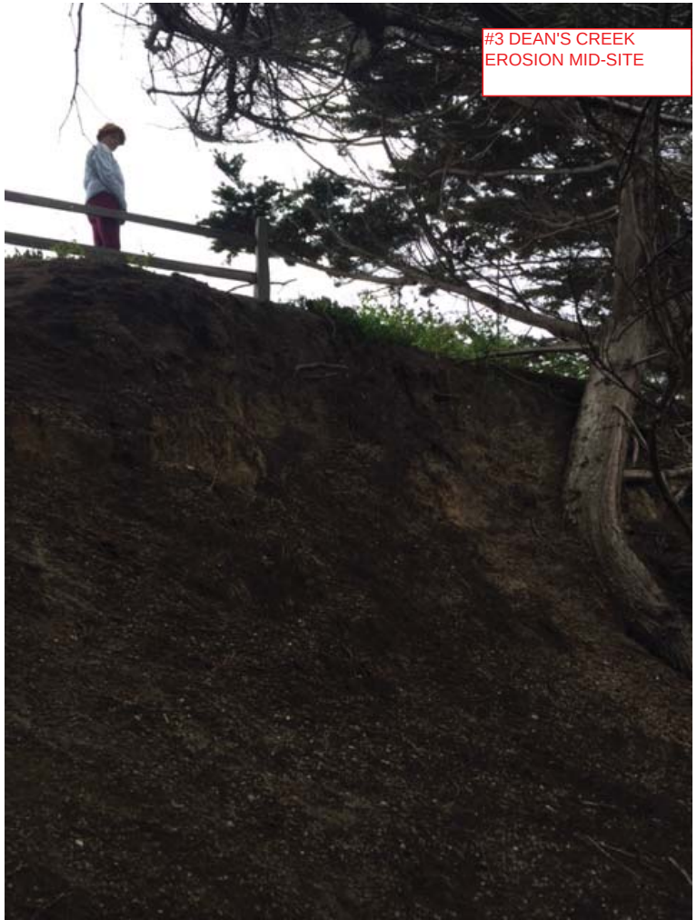
#3 TREE ROOT HOLDING UP DEAN'S CREEK BETWEEN 191 AND 199 ARBOR LANE
