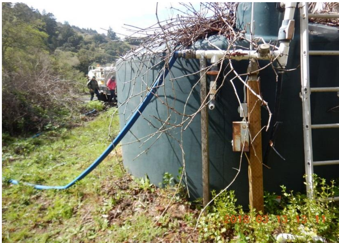
Figure 11. Storage tank associated with Point of Diversion #1.
