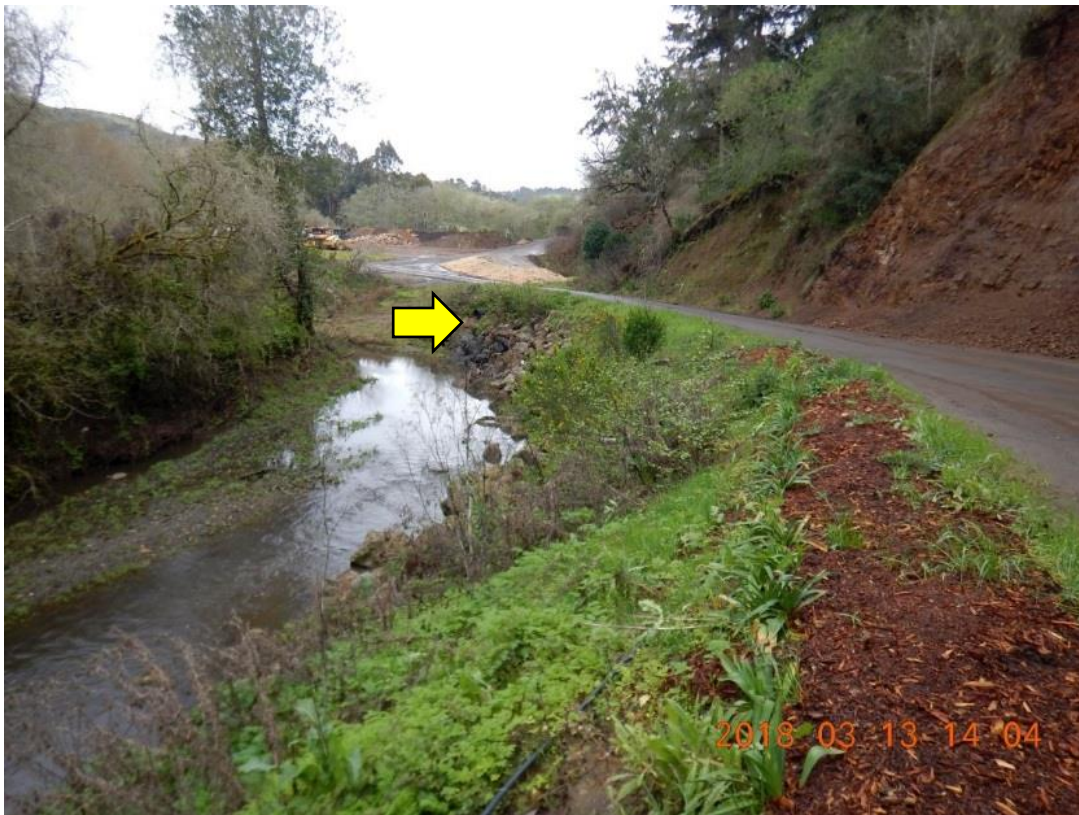
Figure 17. Culvert with associated fill and riprap installed without permits beneath road (also installed without permits) draining swale and emptying into San Gregorio Creek. Yellow arrow indicates location of outfall.
