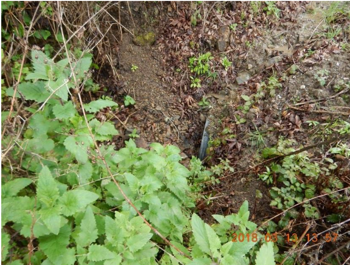
Figure 18. Eastern end of culvert draining swale and road areas, almost entirely clogged by sediment.
