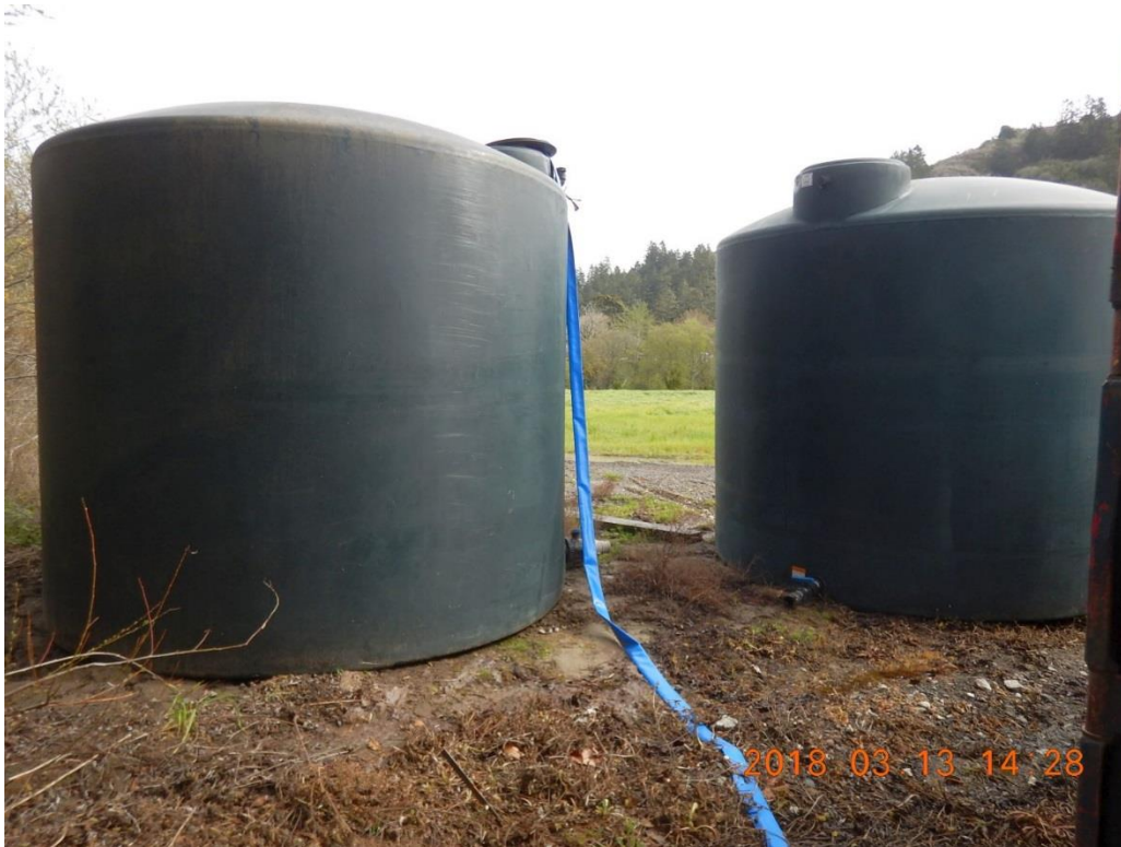
Figure 19. Two 5,000 gallon storage tanks at Point of Diversion #2.
