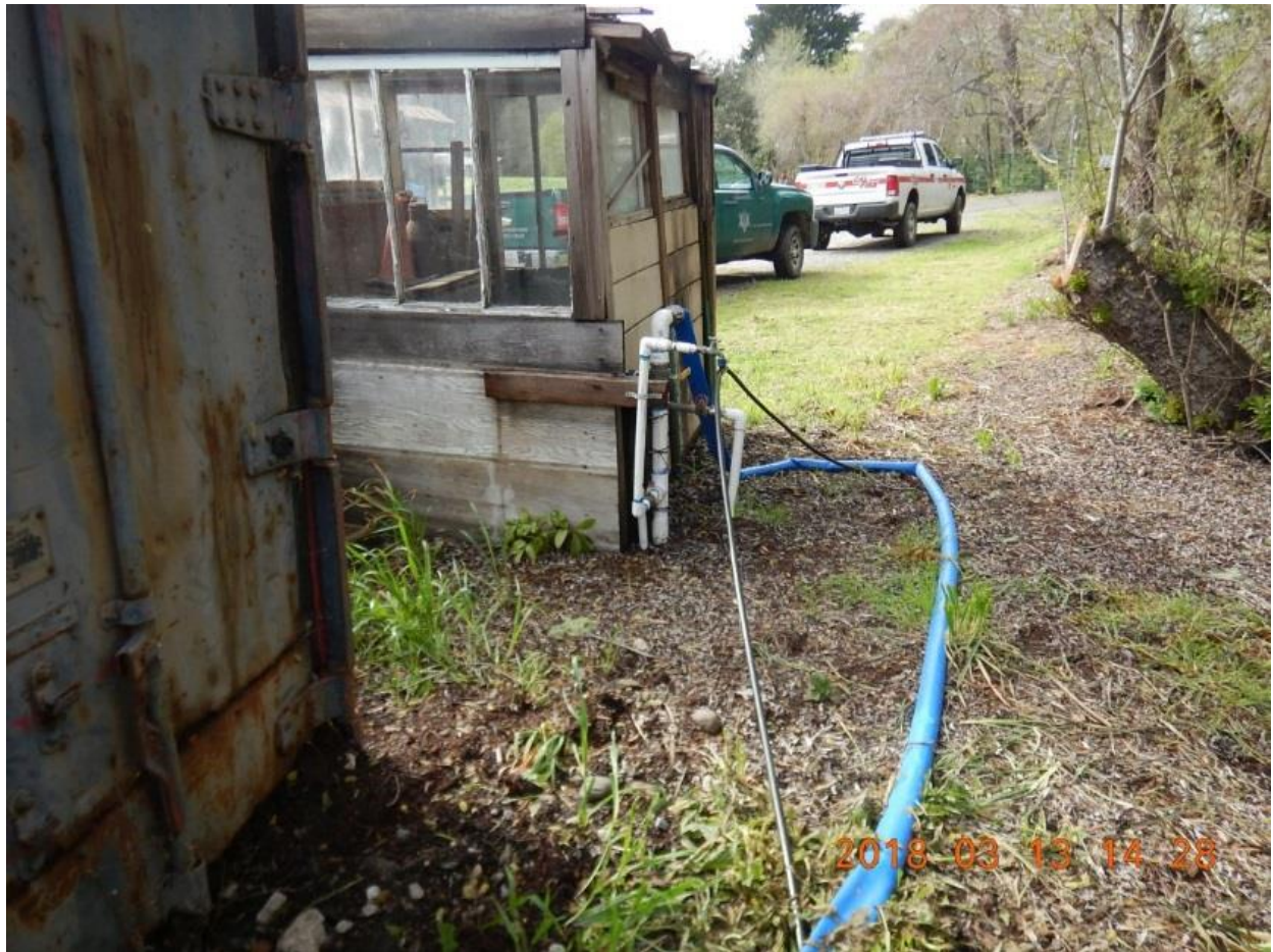
Figure 20. Pump house and hose associated with Point of Diversion #2.
