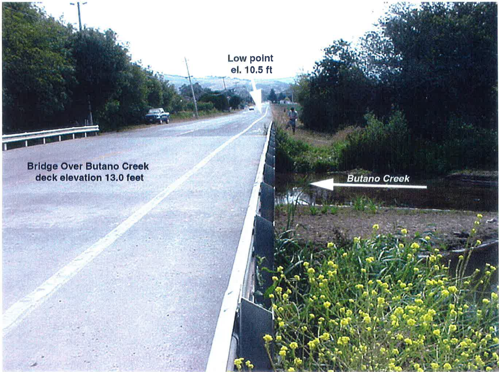
FIGURE 4: PESCADERO CREEK ROAD AND BRIDGE AT BUTANO CREEK LOOKING EAST TOWARD LOW POINT. Photo Date: July 14, 1999
