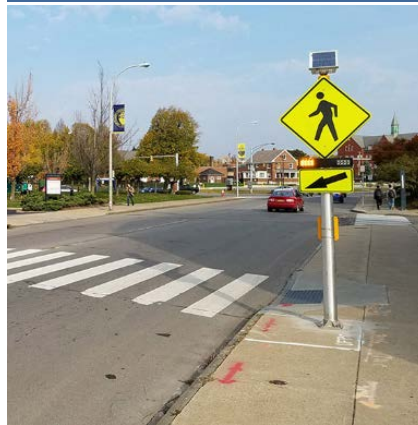
Rapid Rectangular Flashing Beacon
