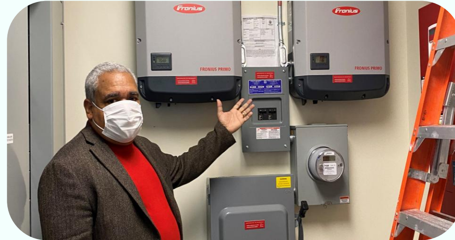
Backup battery system at a church in SSF
