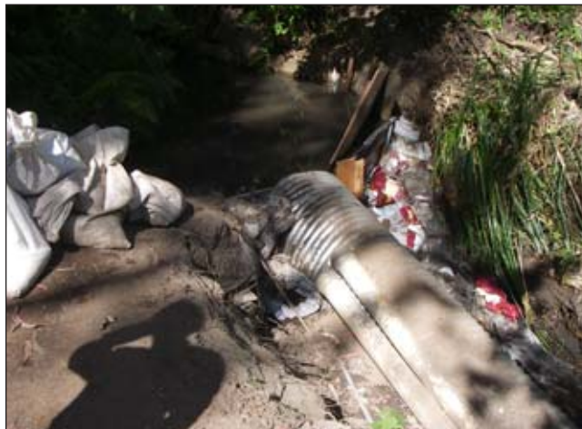
PHOTO 11: Point of Diversion on San Vicente Creek.
