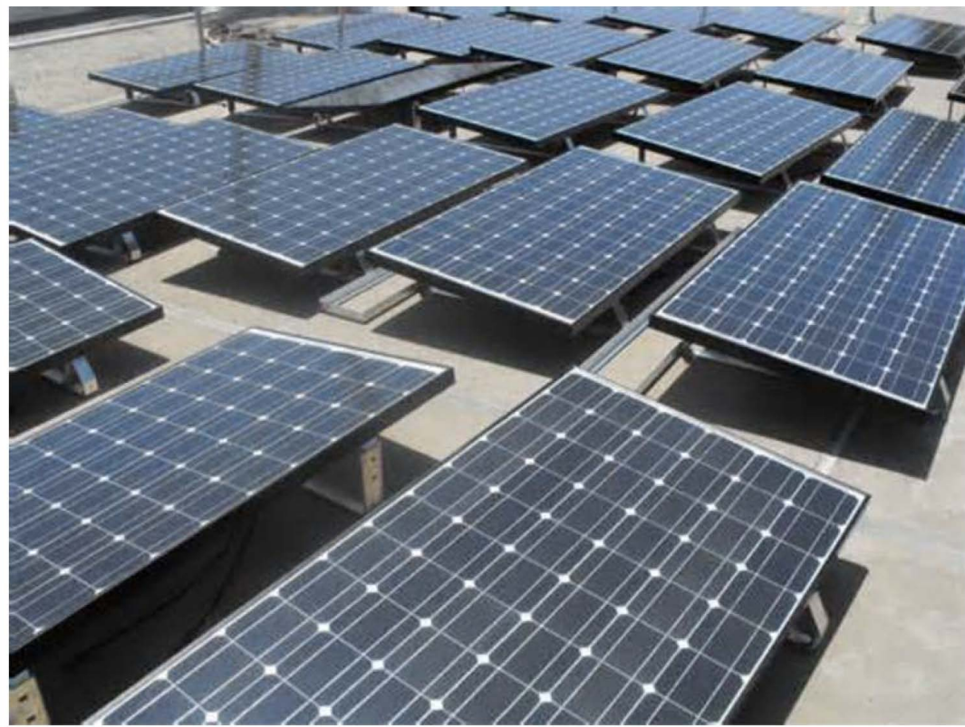
Rooftop Solar Panels
