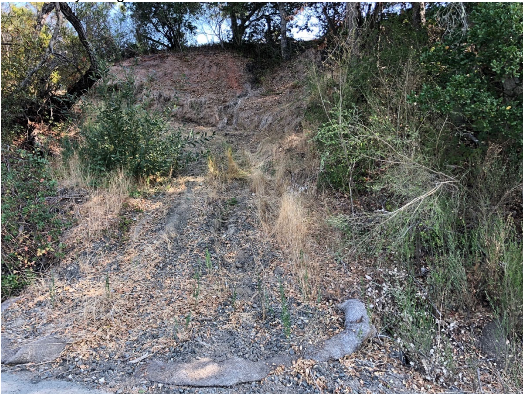
Photo 4. Base of driveway where it meets SR 84/La Honda Road. Straw wattles at base of the driveway where 12" plastic culvert was installed.
