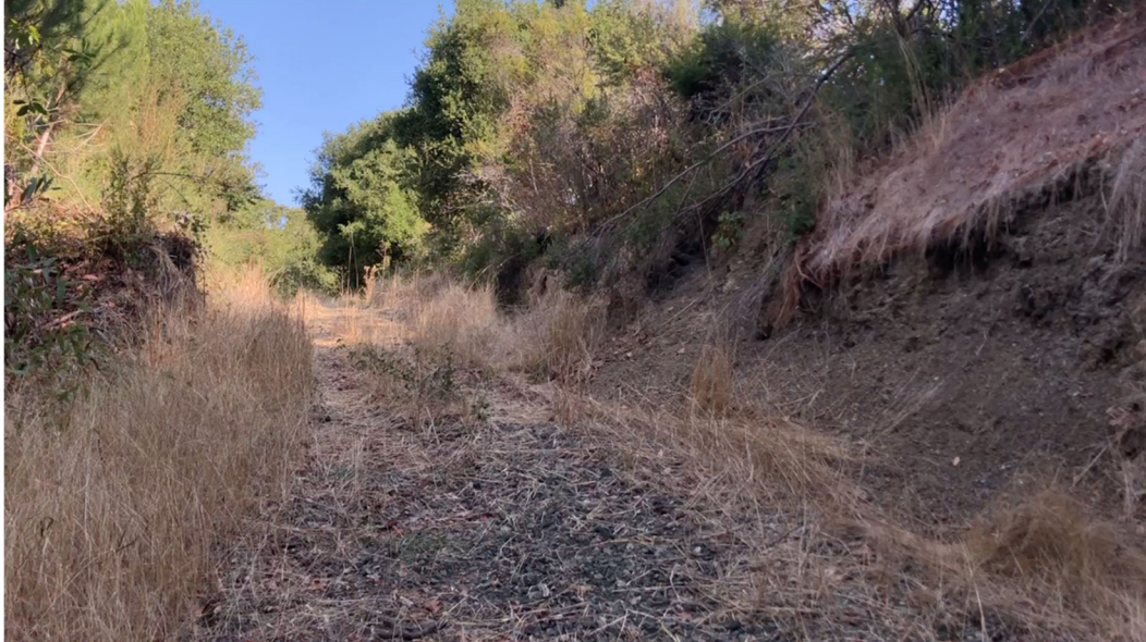
Photo 1. North facing portion of driveway above steep graded turn. Orange plastic netting over eroded slope visible on northeast side.
