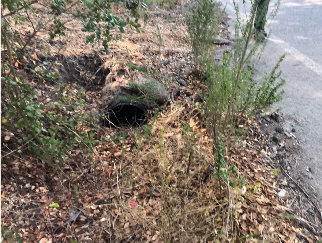
Photo 5. Drainage ditch with 12" plastic culvert at the base of driveway adjacent to SR 84/La Honda Road.
