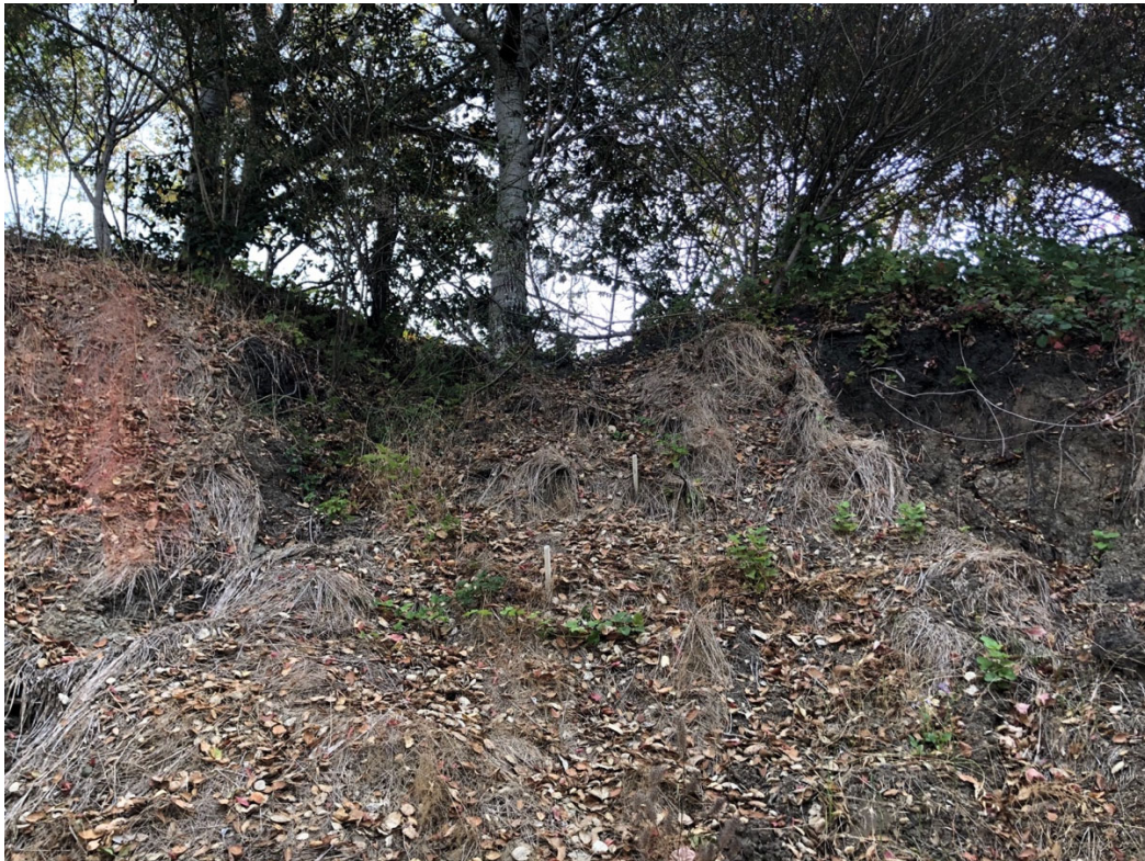
Photo 2. East facing upper slope above driveway. Orange plastic netting over eroded slope visible on east side.
