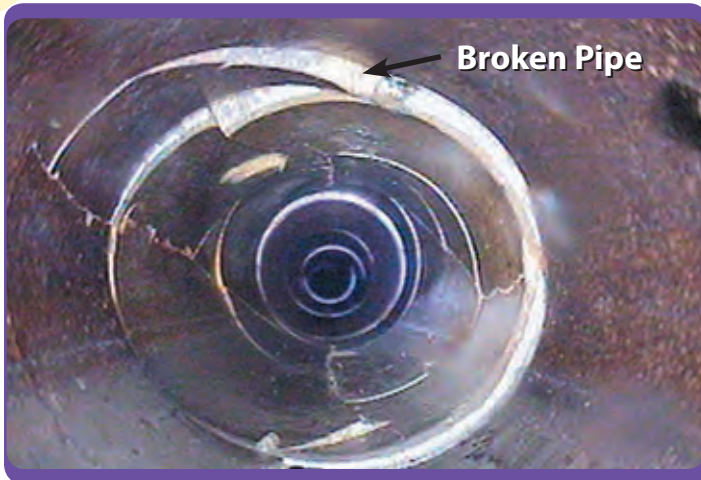
Image #8 – Broken pipe
