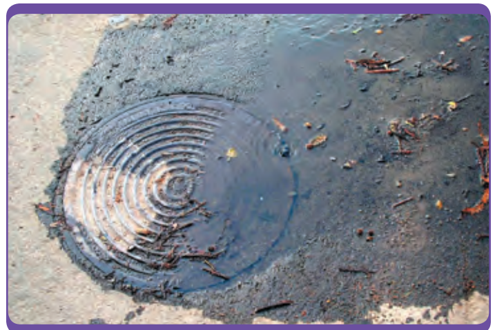
Image #10 – Sewer overflow at sewer manhole
