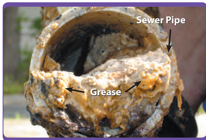
Image #3 – Grease inside of sewer pipe
