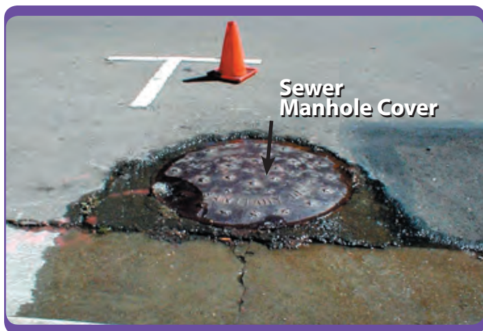
Image #2 – Wastewater flowing out of a sewer manhole cover
