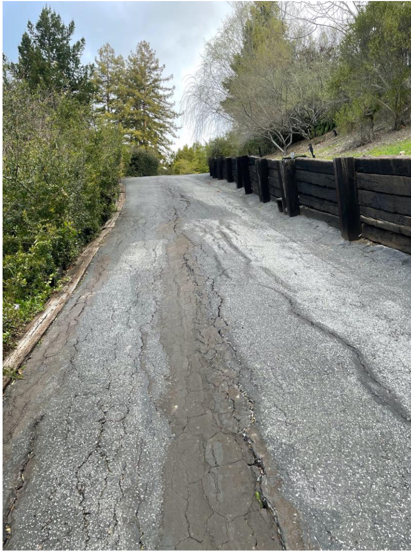
Photo 2 — Looking north and upslope the entrance at 10707 La Honda Road, Woodside, CA 94062 (San Mateo County) (Assessor's Parcel 078-190-210), the wood retaining wall (right side of photo) will be replaced after the driveway is widened as part of the Project.
