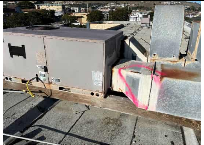
22. View of Duct Seam Mastic and Tape
