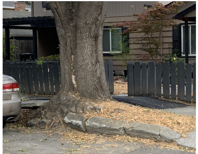
Tree roots uplifted sidewalk and curb. Drainage is affected and ponding could occur.
