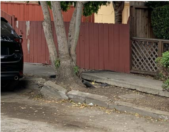
Tree roots uplifted sidewalk and curb. Drainage is affected and ponding could occur.
