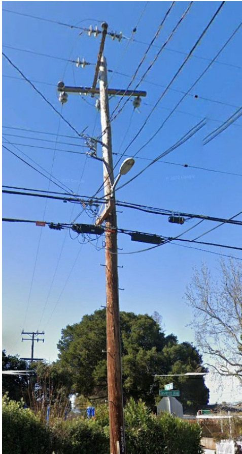
Pole with not enough clearance
