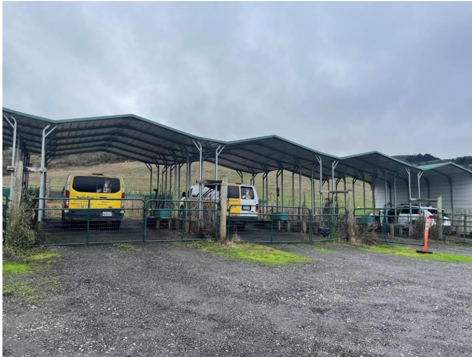
Figure B-1. Covered parking structure for Smilin' Dogs Dog Ranch. Photo date: 12/28/2024.
