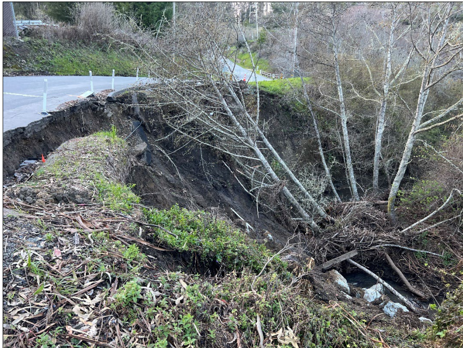
Photo 2: West-facing view of the slip-out area. The photo was taken on March 8 th , 2023.
