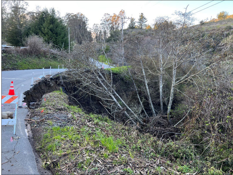
Photo 1: Northwest-facing view of the slip-out area. The photo was taken on March 8 th , 2023.
