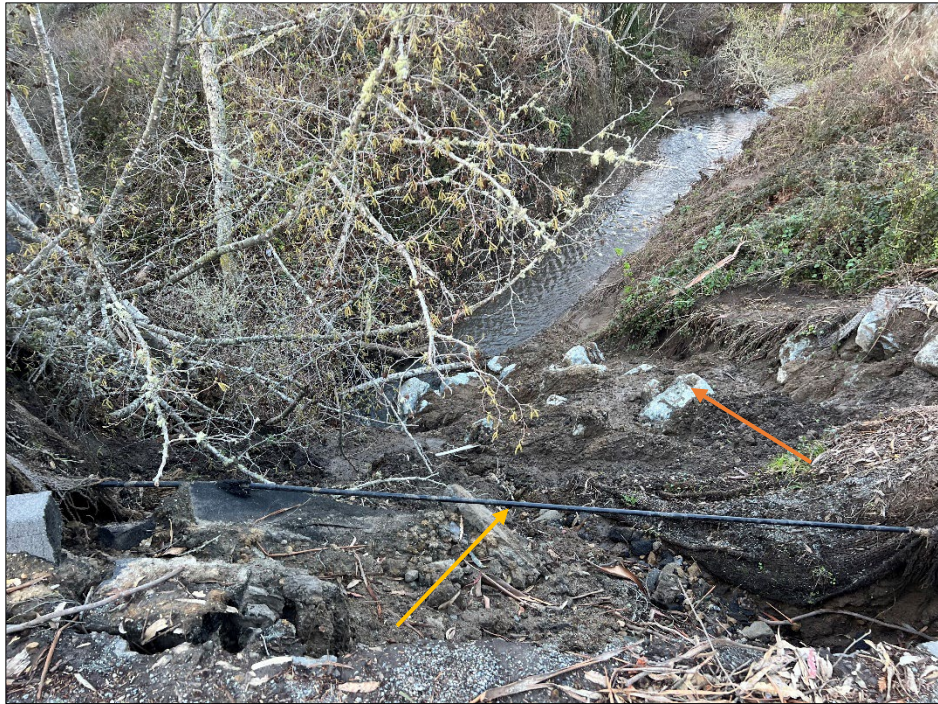
Photo 5: Northeast-facing view of the slip-out area. Note the exposed utility line (see yellow arrow). Also note exposed riprap in slope fill (orange arrow). The photo was taken on March 8 th , 2023.
