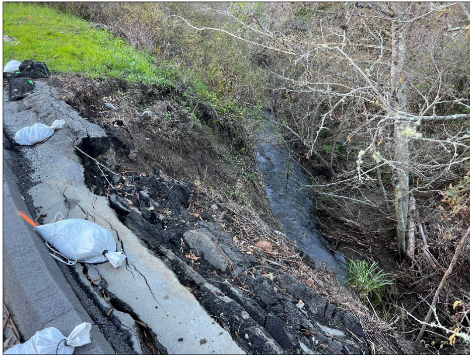
Photo 8: Northwest-facing view of the slip-out area. The photo was taken on March 8 th , 2023.
