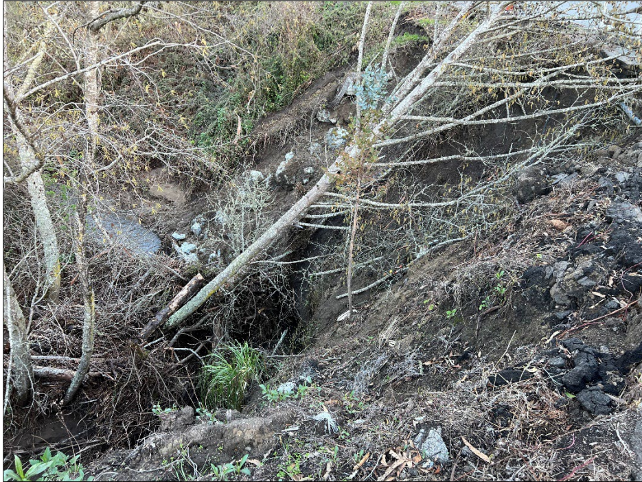
Photo 7: East-facing view of the slip-out area. The photo was taken on March 8 th , 2023.
