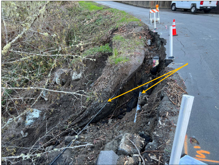
Photo 4: East-facing view of the slip-out area. Note the two exposed utility lines in the scarp area. The photo was taken on March 8 th , 2023.
