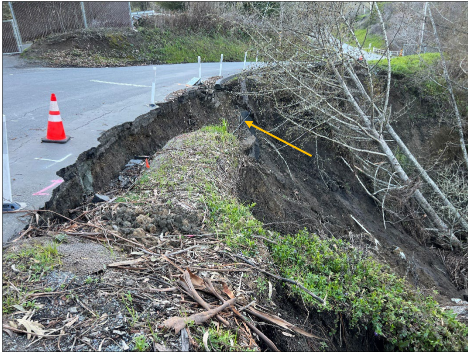
Photo 3: West-facing view of the slip-out area. Note the two exposed utility lines in the scarp area (see yellow arrow). The photo was taken on March 8 th , 2023.
