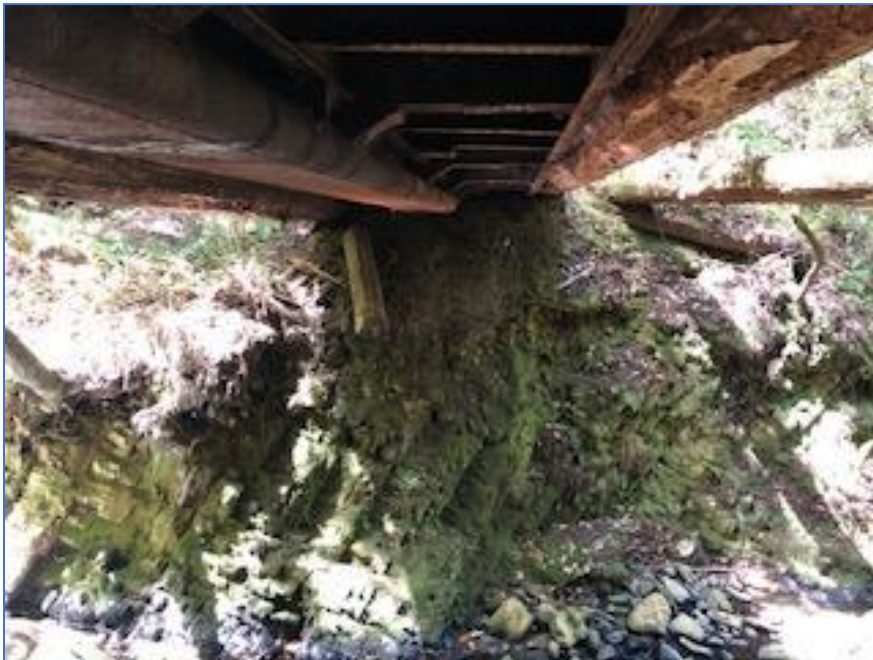
View 4. View of underside of existing bridge, showing old railroad car understructure.
