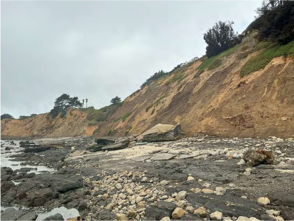
Photo 5: Collapsed foundation, originally atop the sea bluff, now along the beach between San Lucas Avenue and La Grande Avenue. Photo taken facing north. Date of photo: July 27, 2025.
