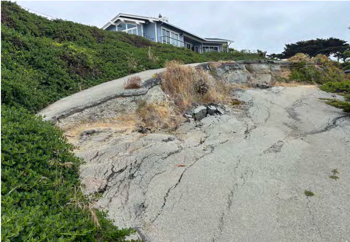
Photo 2: Scarp at the intersection of La Grande Avenue and Ocean Boulevard. Photo is taken facing southeast. Height of the scarp is 4-6 feet, with the downslope side facing the sea bluff. The asphalt above the scarp is sloped inland. Date of photo: June 25, 2025
