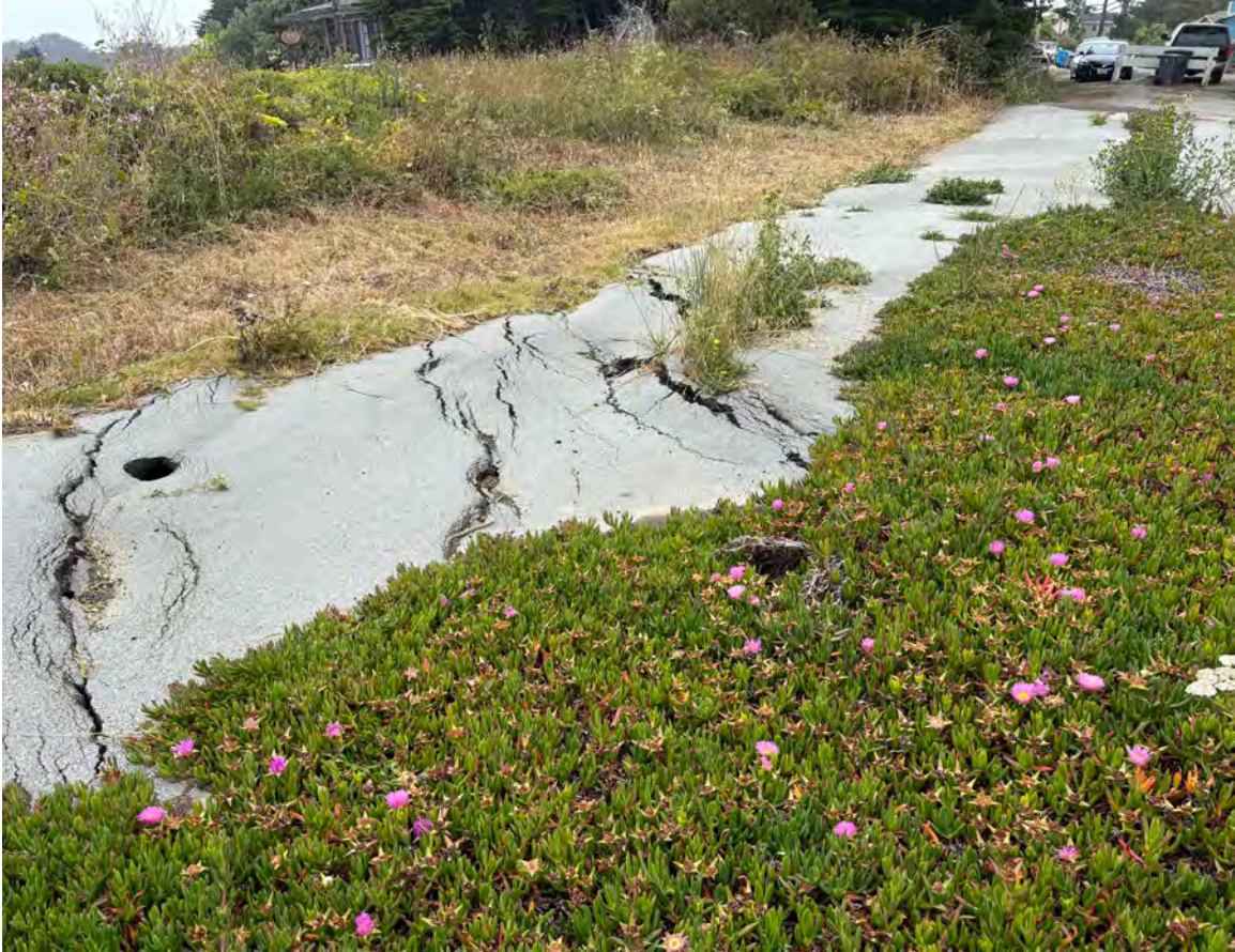
Photo 4: Graben, cracking, and sink hole (left) along San Lucas Avenue between Ocean Boulevard and Del Mar Avenue. Photo taken facing north. Date of photo: June 25, 2025.
