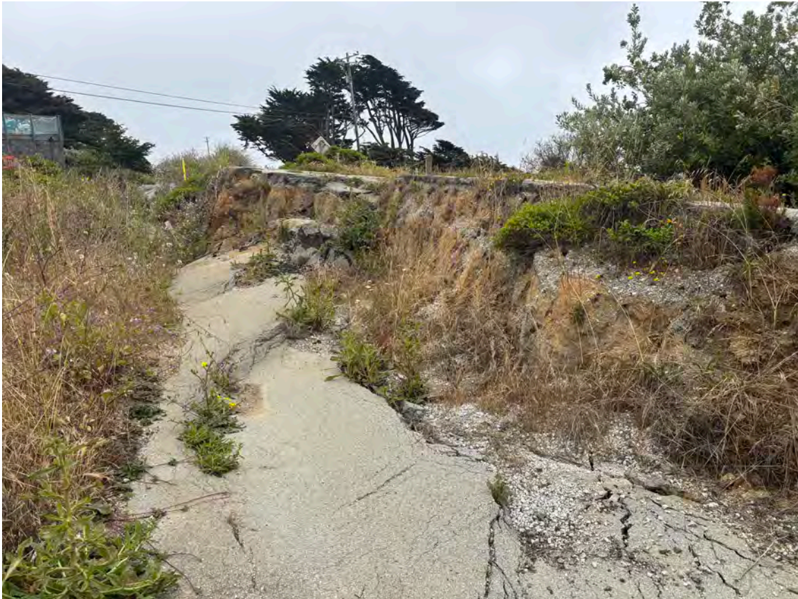
Photo 1: Scarp along Ocean Boulevard, between San Lucas Avenue and La Grande Avenue. Photo is taken facing toward the south. Height of scarp is 3-7 feet, with the downslope side facing inland (away from the sea bluff). Date of Photo: June 25, 2025
