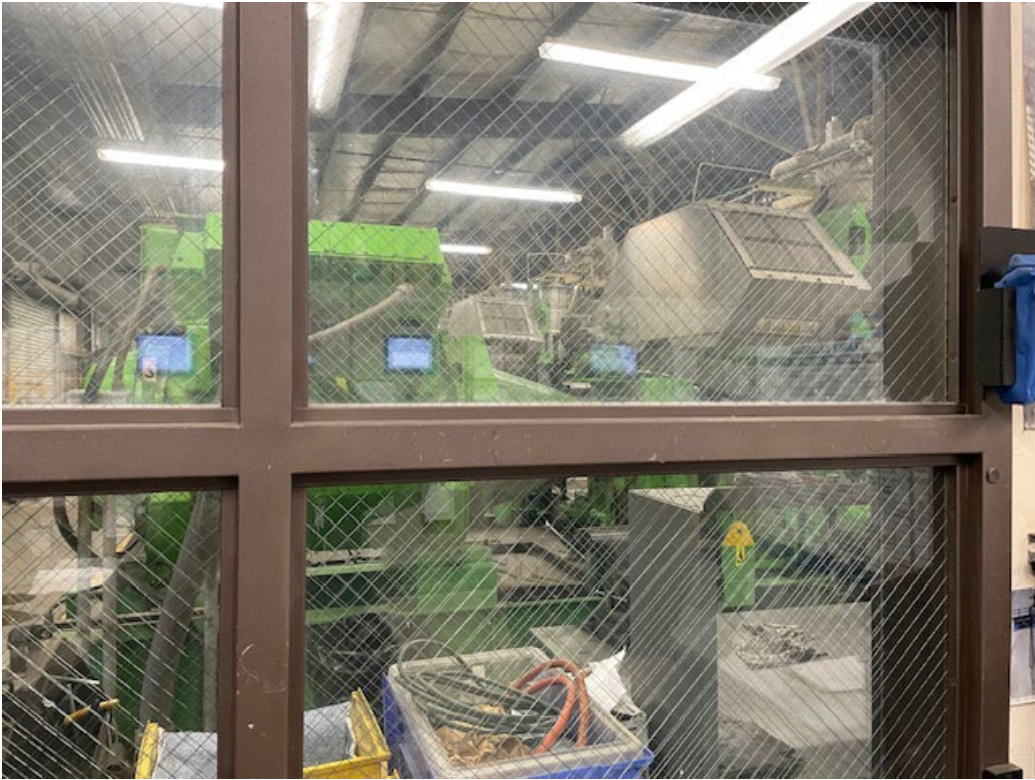
Figure 4 - View of Jenbacher Landfill Gas Engine Generators inside the Ameresco plant building
