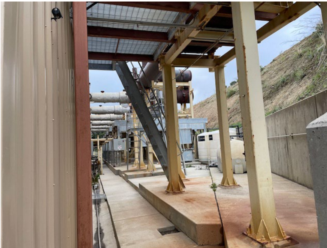
Figure 6 – Exhaust and radiator area behind the Ameresco Plant Building
