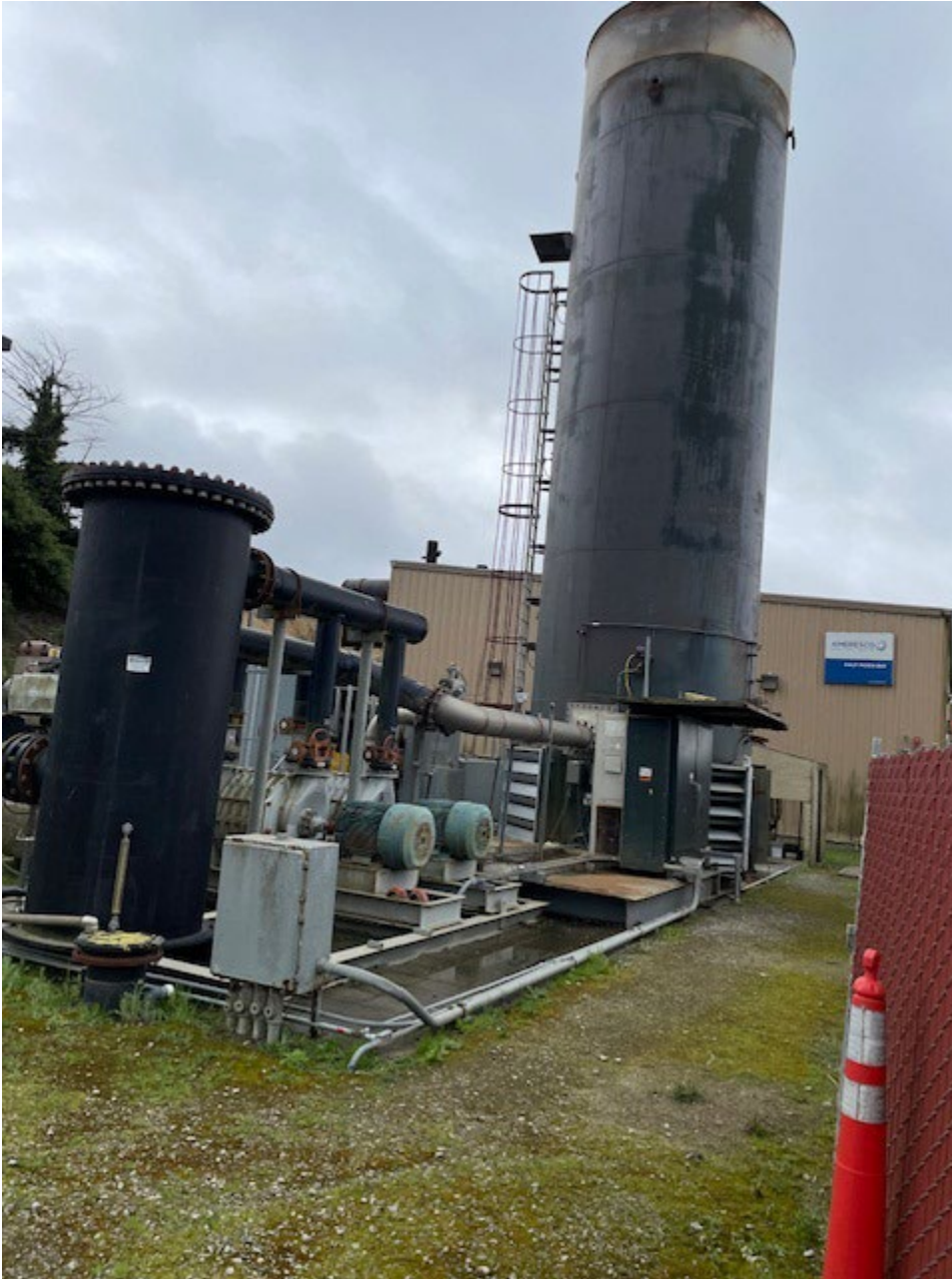
Figure 7 – Republic Landfill Gas Flare which is used when the Ameresco Plant is not operating to combust the landfill gas from the landfill wellfield.
