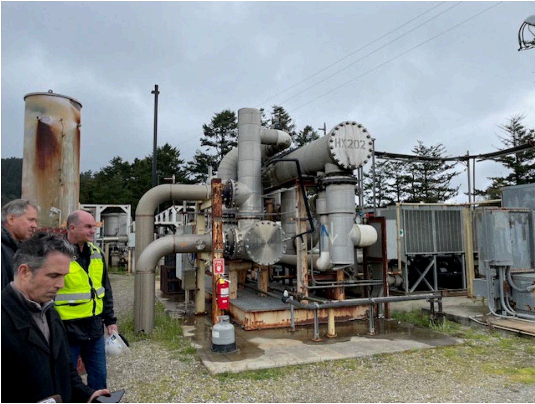
Figure 8 - Ameresco Gas Cooling Skid
