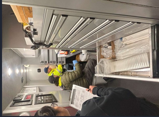
1030 Commercial St. San Carlos HazMat
