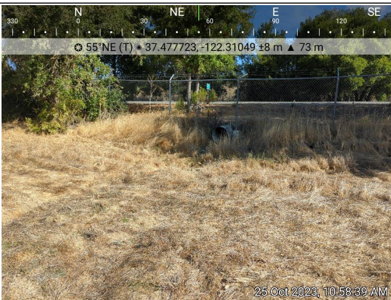
Photo 4. One of two outfalls occurring beneath Cañada Road. Both drainages currently have overland runoff feeding nearby creeks. Development of channels feeding a retention basin is proposed within the current project scope.
