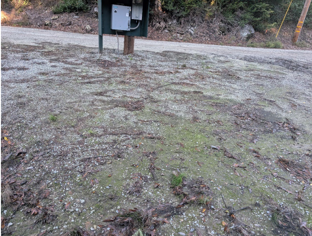
Photo 3. Wellfield & Pilarcitos Creek Road
