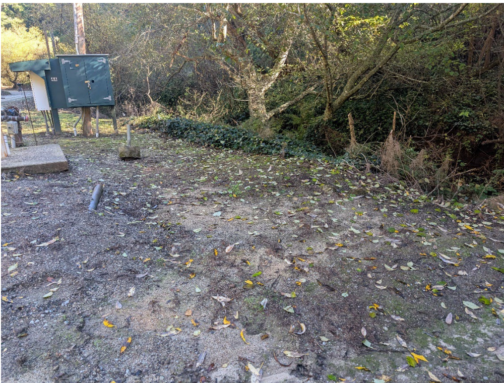
Photo 8. Pilarcitos Creek Wellfield
