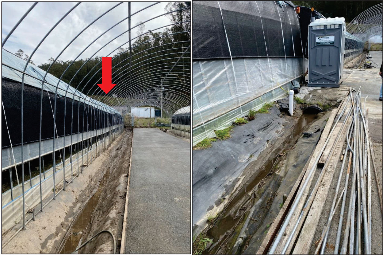
Figure 9. A concrete and geotextile-lined modified tributary adjacent to a mushroom building (left and right picture, PL-1). The reservoir embankment is visible in the background (red arrow in left picture).
