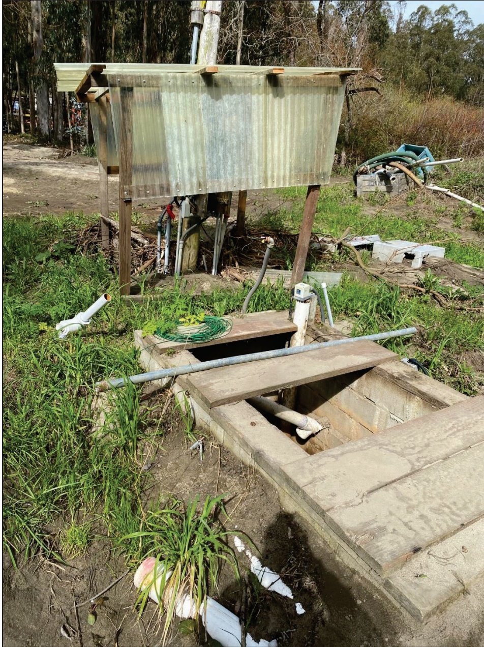
Figure 3. Steep-walled hole or pit next to the water diversion system (WS-1).
