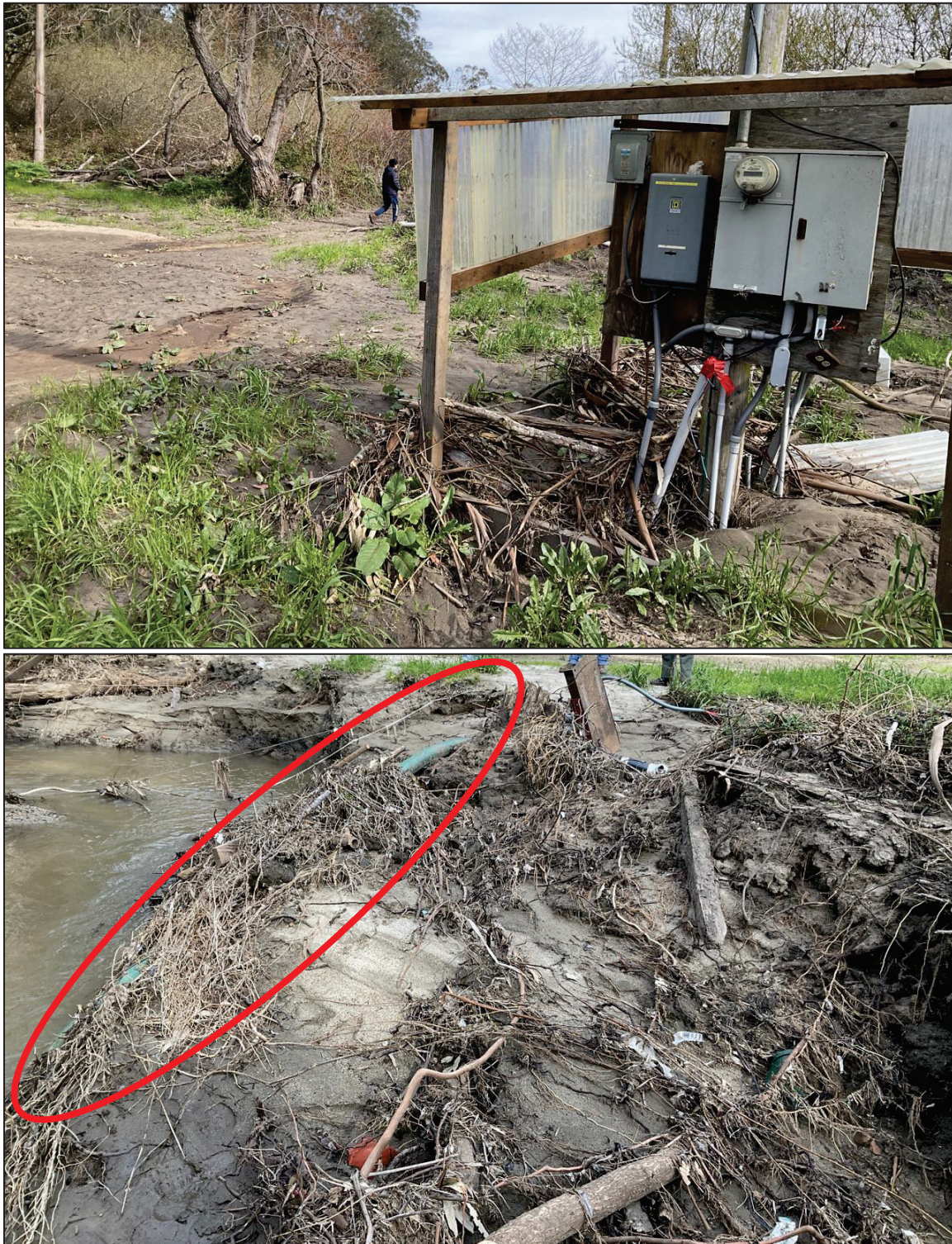
Figure 2. View of debris located at WS-1 includes an electrical panel within 150 feet of
