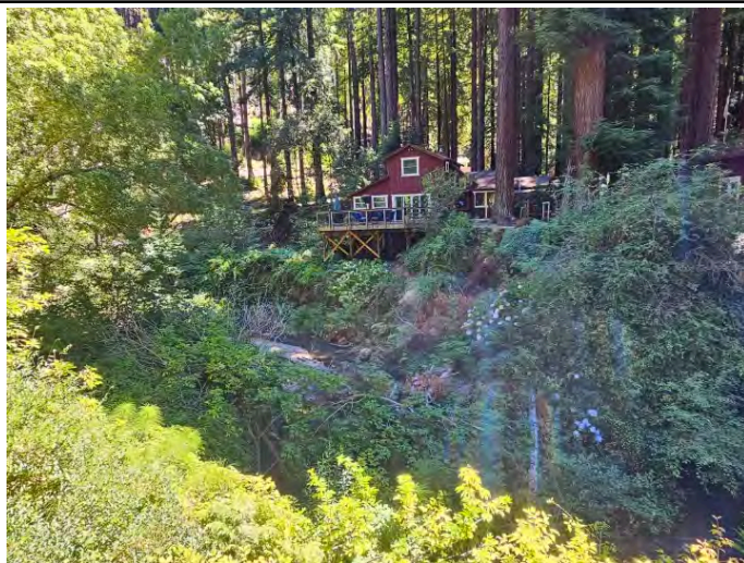
BEFORE (2024): View of eroded bank beneath home. Taken from neighbor's property looking towards house.
