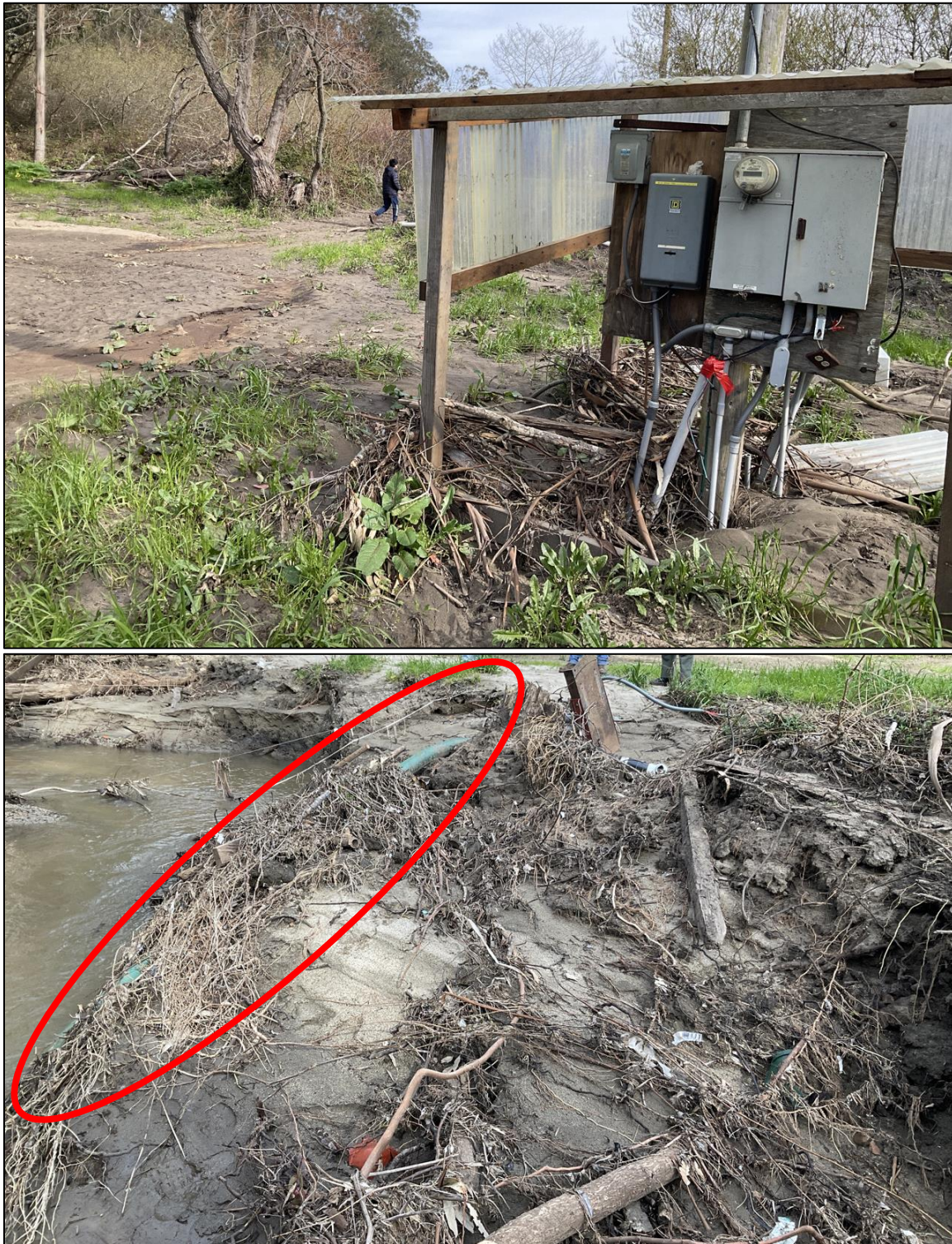
Figure 2. View of debris located at WS-1 includes an electrical panel within 150 feet of
