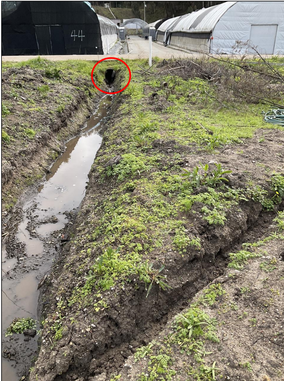
Figure 10. A 26-inch corrugated metal pipe (red circle, SC-1) marks the transition to a modified tributary that flows to Pilarcitos Creek.
