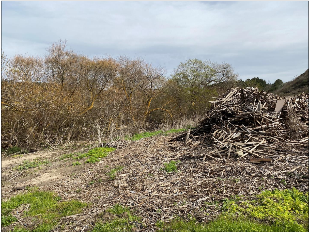
Figure 12. Wooden debris from a demolished building at PP-3 within 150 feet of Pilarcitos Creek.
