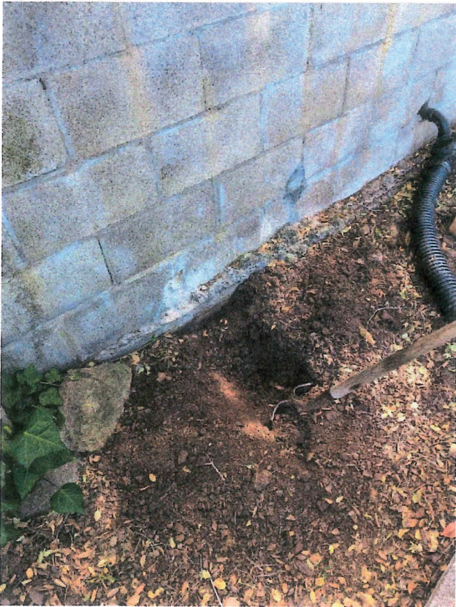
Photo 2 – Embedded shovel showing extent of concrete footing below
