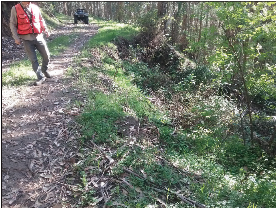
Figure 2: Fillslope failure on the South Ridge Vista Trail.
