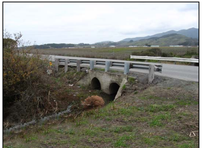
View 5: Along Airport Street, the roadway culvert identifies the drainage area that separates the project parcels. Half Moon Bay Airport facilities are visible in the background.
